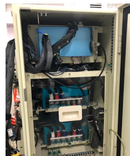
Photo of rack installation
